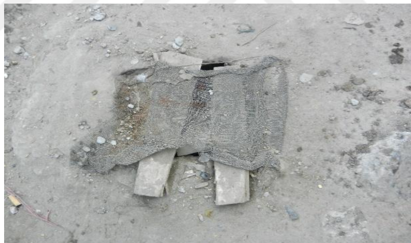
Figure 8. Drainage issues on the site Source: Yazdaan Hiader Khan
