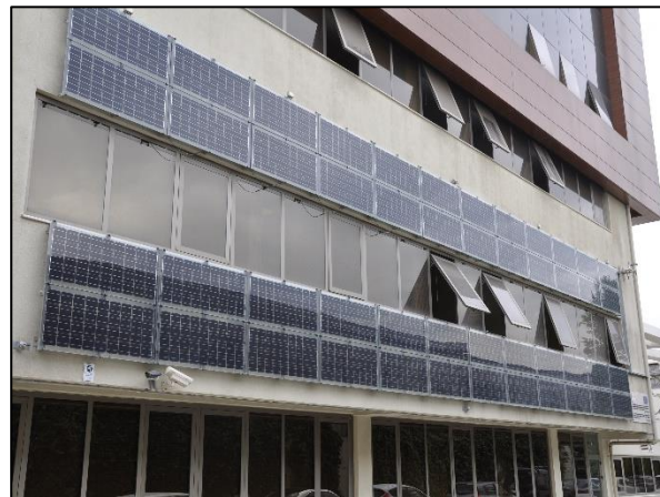
Figure 2.5. The BIPV system at Yaşar University, Izmir, TURKEY.
